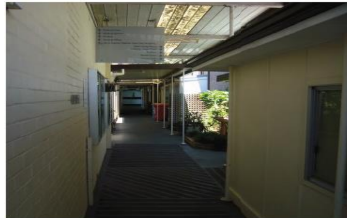
4. Inappropriate access arrangements between buildings
