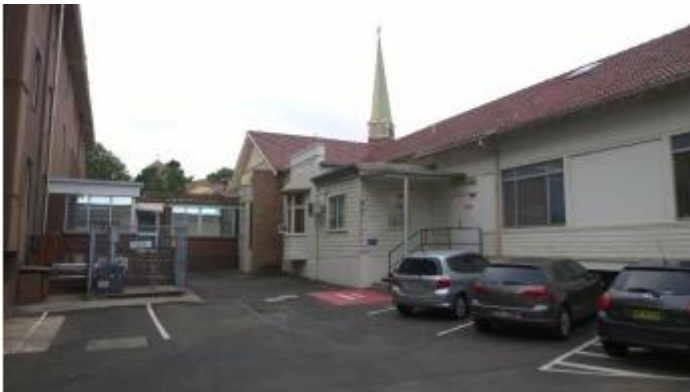
3. Ambulatory Care services building is past functional life – built 1952 (inpatient palliative care building also built 1952)
