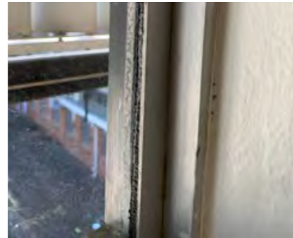
Seals/caulking to external windows crumbling.
