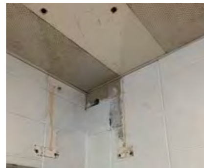
Ceiling dirty and walls require patching and painting.
