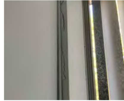
Cracks in walls. Structural review recommended
