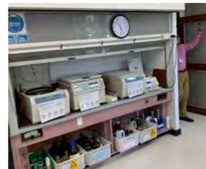
Obsolete fume cupboards.
