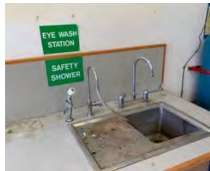
Generally eye wash units are non-compliant to current standards.
