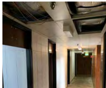
Dirty and damaged ceilings
