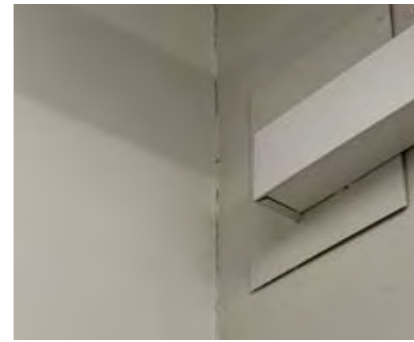
Some cracks noted in wall junctions.
