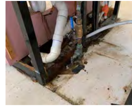
Stained vinyl flooring with open joints and sections missing. Exposed timber and pipework which are dirty and not easily cleaned.
