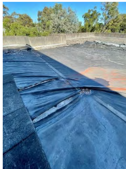
Failure of rooftop membrane
