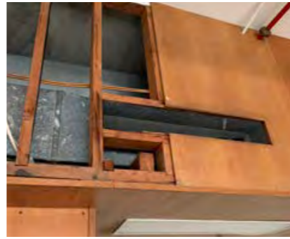
Timber bulkheads in need of repairs
