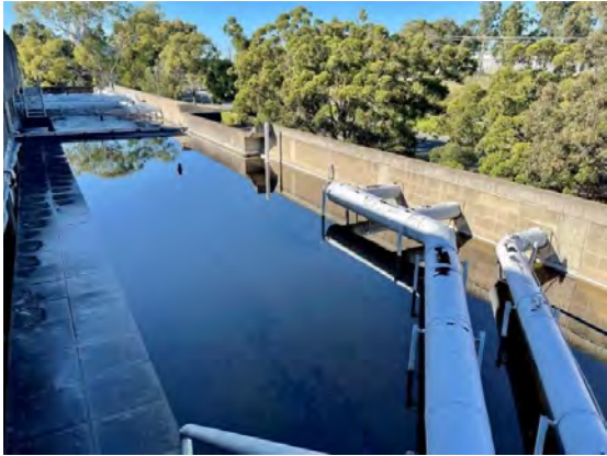
Standing water at roof
