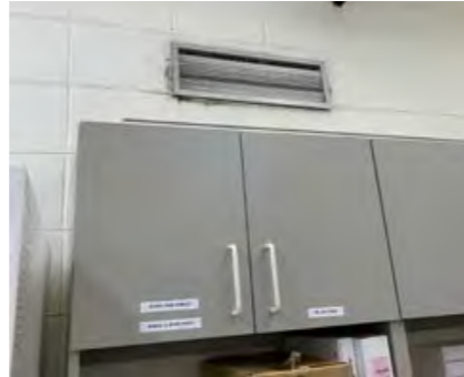
Generally walls not smooth, and timber joinery throughout
