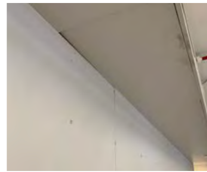
Bulkheads are uneven with gaps at junctions exposing space to ceiling cavity.
