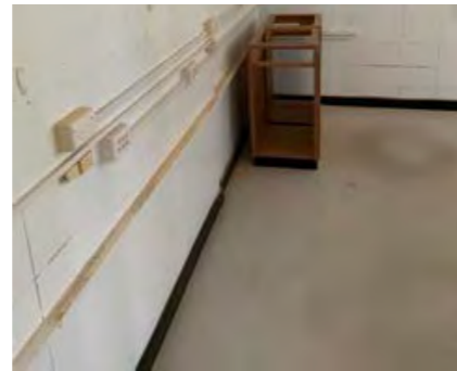
Walls damaged from removal of fixed joinery, skirting etc. Fixings need to be removed and walls patched/painted.
