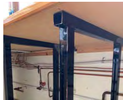
Exposed/unsealed timber under benchtops. Steel hollow section framing have open ends and holes throughout would be impossible to clean out. Exposed surface mounted gas lines and power conduits difficult to clean.
