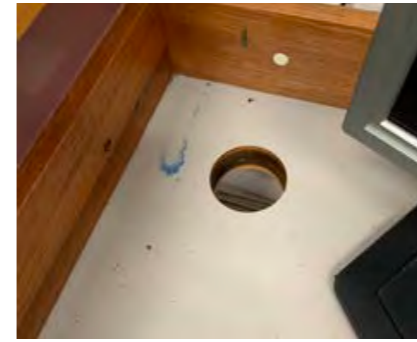
Exposed timber, and benchtop substrate exposed in cutout.
