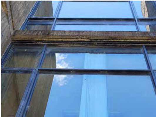
Evidence of likely reinforcement corrosion and concrete spalling
