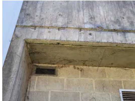
Cracking to loadbearing walls
