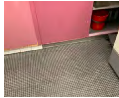
Finish to joinery damaged exposing timber.
