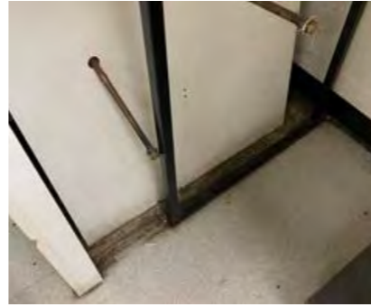
Flooring generally dirty and deteriorating or damaged.
