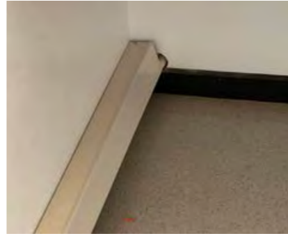
Unsealed penetrations in wall
