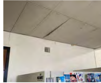
Perforated ceiling tiles difficult to clean and needs to be refitted
