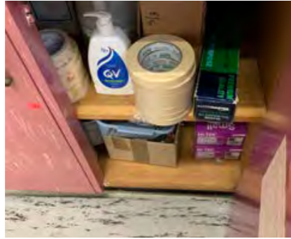
Exposed/ unsealed timber in joinery
