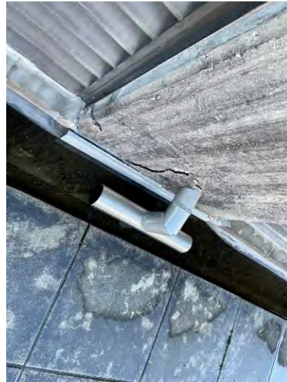
Large cracks at external roof supports
