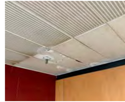
Evidence of water damage to ceiling tiles
