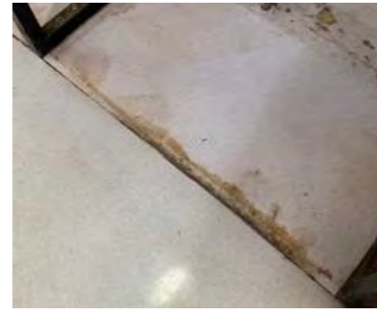
Stained vinyl flooring with open joints.
