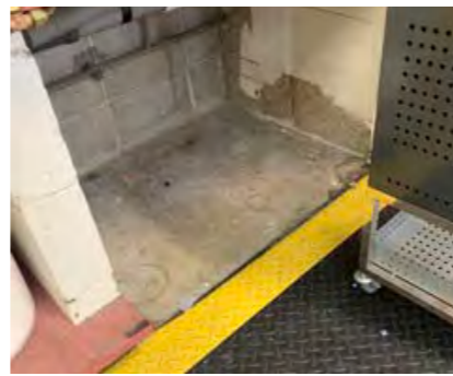
Exposed concrete floor should be sealed, and checker plate flooring difficult to clean.
