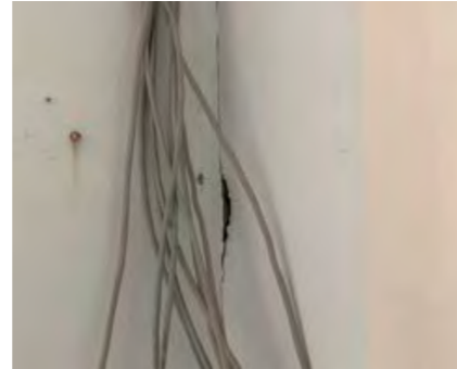
Cracking in corner of masonry wall. Structural review recommended
