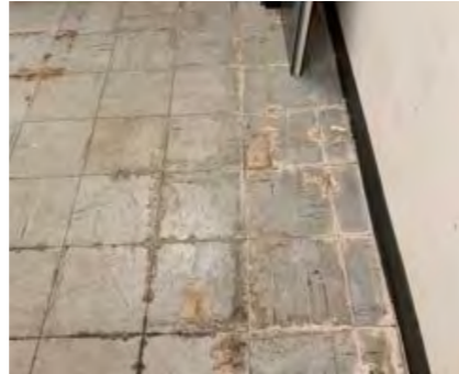
Floor tiles have water damage and staining. Possibly asbestos tiles.
