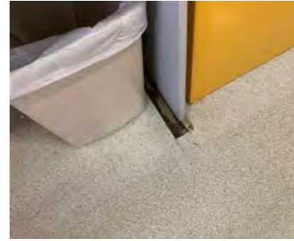
Vinyl flooring damaged/missing and unsealed in areas
