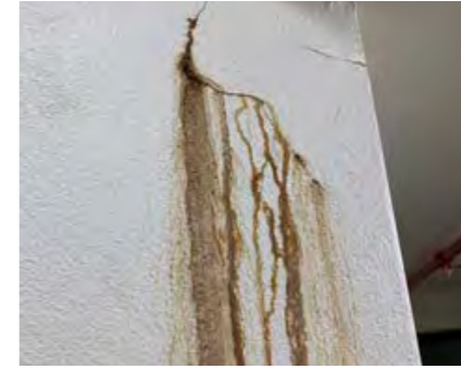
Cracks noted in walls with moisture seepage stains. Appears to be recent, and could be cause of staining on floors.
