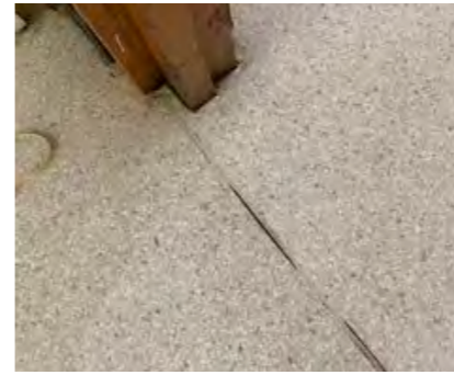
Welded joints in vinyl flooring failing exposing gaps.
