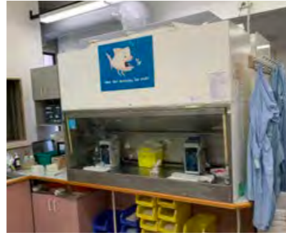
Fume cupboard may be obsolete and no longer usable.
