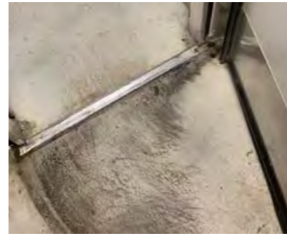
Floor/threshold to freezer door dirty
