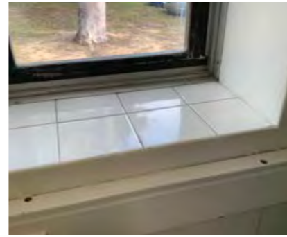
Similar issues with crumbling seals to external windows and tiled sills.
