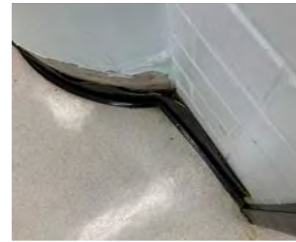
Damaged skirting and wall finishes.
