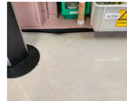
Vinyl flooring lifting in areas.
