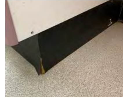
Damaged finish to joinery bases
