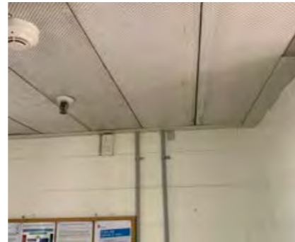
Old and dirty ceilings
