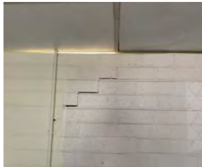
Noted cracks in walls suggesting some movement in structure.
