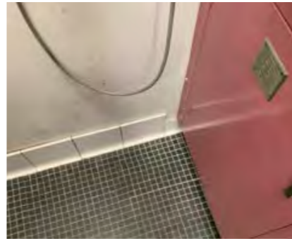
Tiled floor and skirting would be difficult to clean. Skirting tiles pulling away from walls
