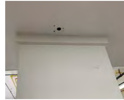
Penetrations not sealed, exposing bulkhead cavity to lab space.
