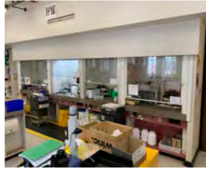
Fume cupboards appear to be obsolete and not fit for purpose.
