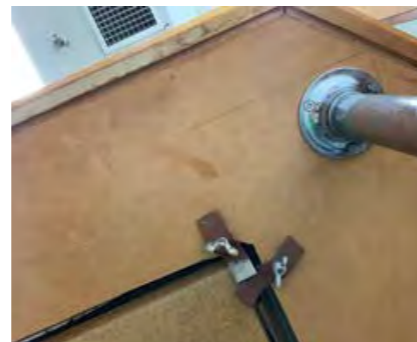
Timber joinery generally throughout labs with exposed/unsealed timber.
