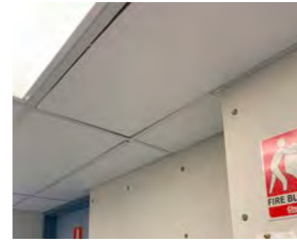
Ceiling tiles are smooth and generally well fitted. Observed some tiles that have gaps to grid and require to be refitted, and also edges of tiles are not sealed.
