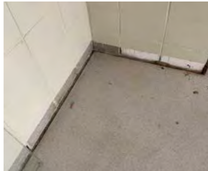
Open gaps between wall and flooring
