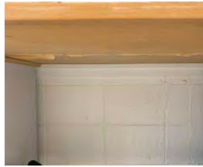
Generally walls not smooth or easily cleanable. Exposed timber under benchtops.
