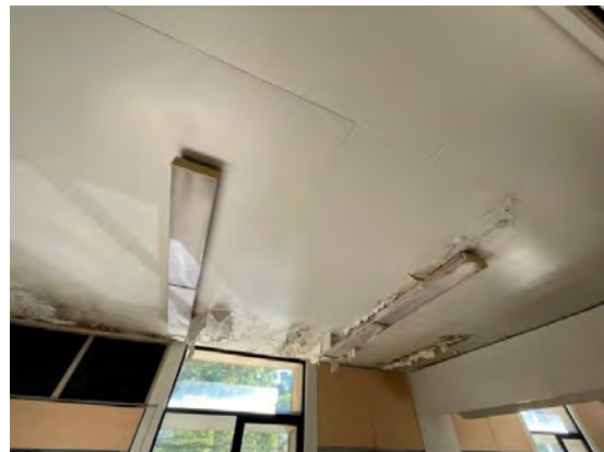
Water ingress through building construction joint
