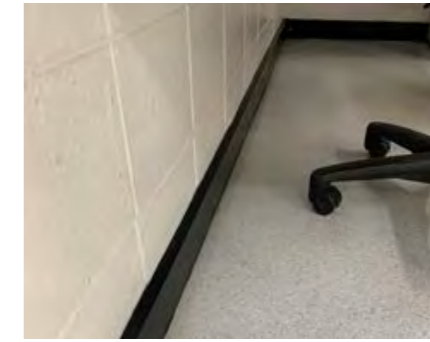
Older vinyl flooring and timber skirting throughout, but appears to be well maintained & clean.
