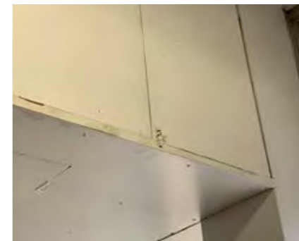
Bulkhead panels with numerous gaps and damaged paint finish exposing timber substrate.
