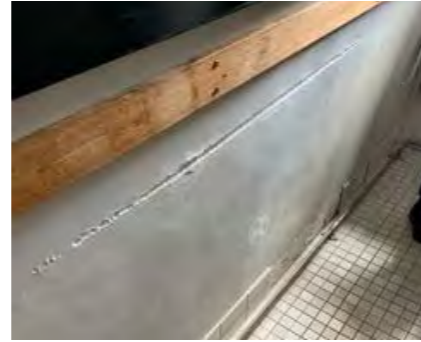
Damaged wall and sections of tiled skirting missing.
