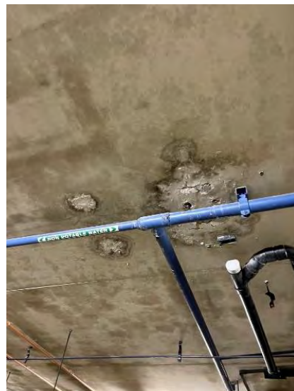
Evidence of likely reinforcement corrosion and concrete spalling at penetrations for services
