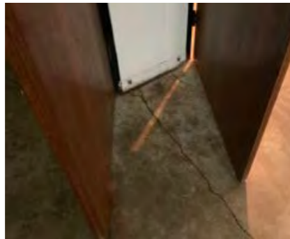
Cracks in concrete floor. Structural review recommended
