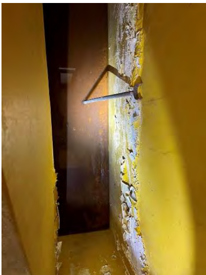
Ponded water throughout
