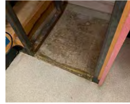
Vinyl flooring missing.
