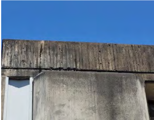
Evidence of likely reinforcement corrosion and concrete spalling at roof slab joint
