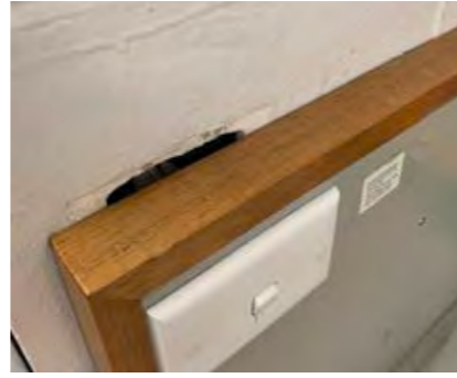
Penetration through blockwork wall not patched/sealed.
