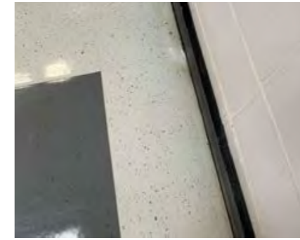
Vinyl Flooring lifting in areas
