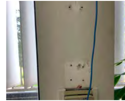
Damaged walls requiring patching and painting
