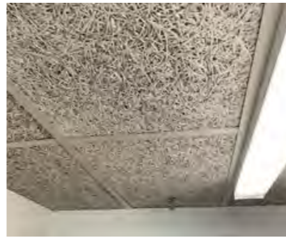
Fibrous straw based ceilings inappropriate for lab spaces
