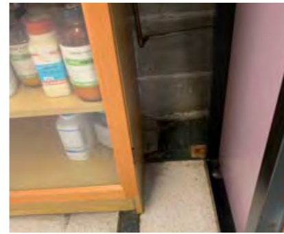
Raw unfinished blockwork in one lab. Possibly in other areas hidden by joinery/furniture
