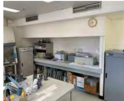
Obsolete fume cupboard no longer functional
