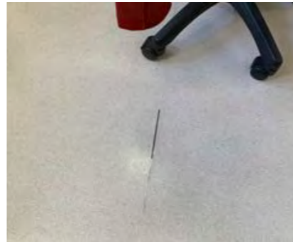
Stained or damaged vinyl flooring in numerous areas.
