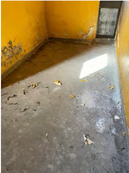
Extensive water damage at concrete joints and linings
