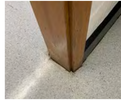
Typical issues with vinyl flooring not sealed at junctions.
