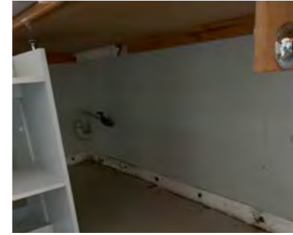
Damaged walls where skirting were removed.
