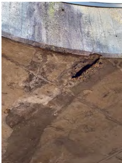
Evidence of likely reinforcement corrosion and concrete spalling in external surfaces
