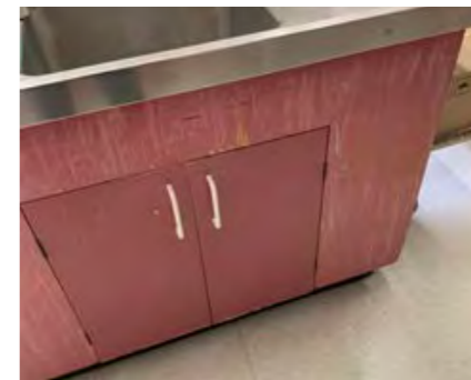
Joinery surface stained and damaged, exposing timber substrate.
