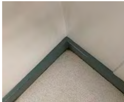
Generally timber skirting with uncovered skirting throughout. Hard to clean.
