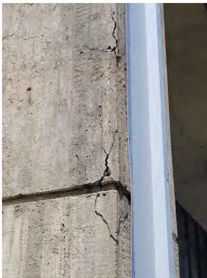
Cracking to external column
