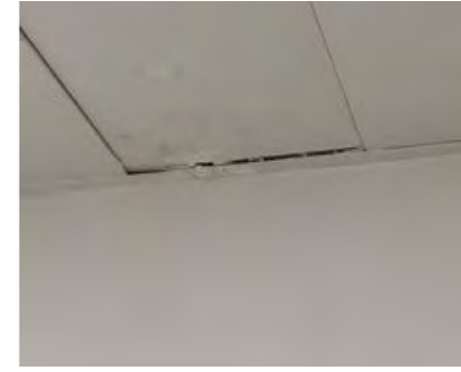
Damaged ceiling tiles
