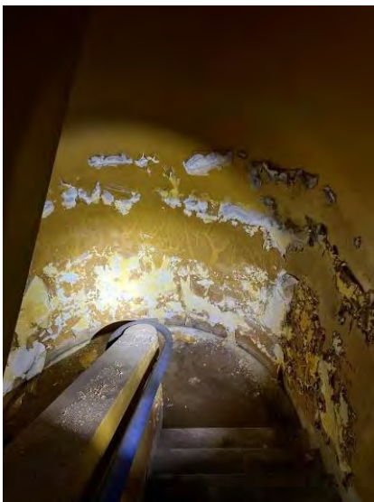
Water damage to stair cores
