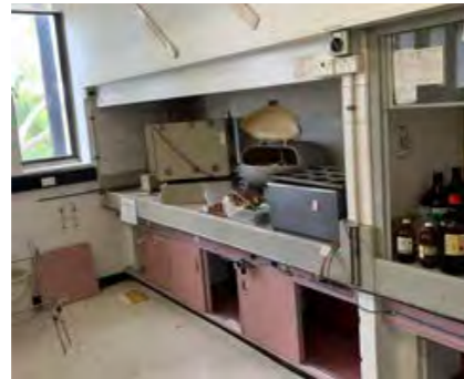
Fume cupboards appear to be non-compliant or functional.
