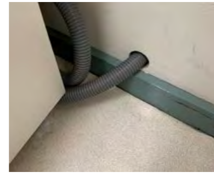
Wall penetration not sealed.
