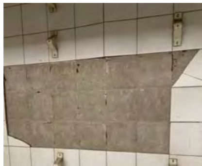
Damaged tiled splashback
