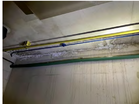
Water ingress through building construction joint
