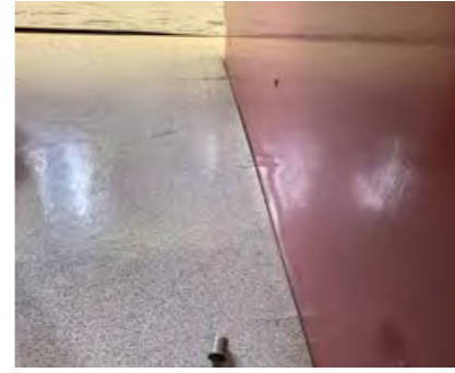
Vinyl flooring in poor condition and lifting off surface
