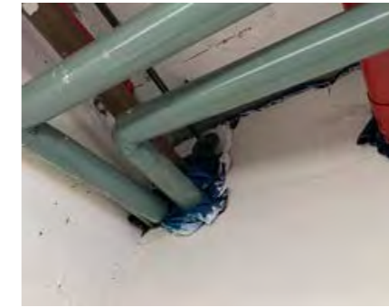
Penetrations through wall generally untidy and not appropriately sealed.
