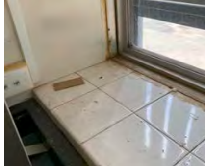
Tiled sill difficult to clean. Window frame needs to be sealed to adjoining surfaces. Caulking to glass crumbling.
