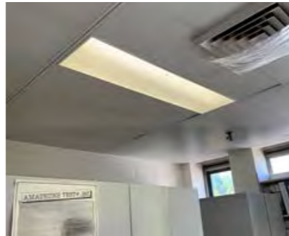
Perforated metal tiled ceiling are generally dirty and backing may be compromised exposing space to contaminants from ceiling space. Needs further investigation to confirm risks.
