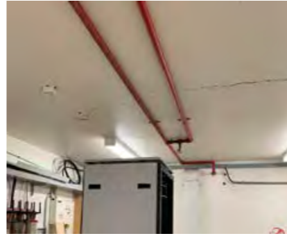
Cracks noted in concrete soffit.
