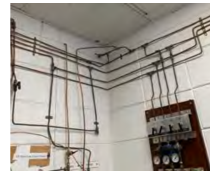
Surface mounted gas lines difficult to clean, and not adequately labelled s a safety concern.
