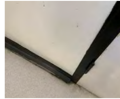
Timber skirting generally need repairs or replacement. Coved skirting would be preferred throughout.
