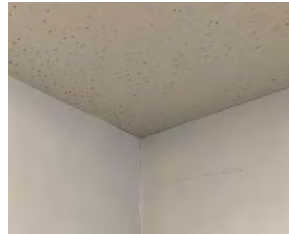
Horizontal and vertical cracks in corners of rendered walls. Recommend structural assessment.
