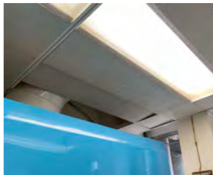
Retrofitted fume cupboard exhaust has exposed ceiling cavity to room.
