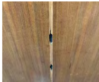
Timber panels in corridor damaged.
