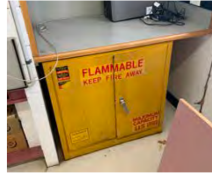
Noted number of flammable cabinets throughout laboratory. They don't appear to be vented. Further investigation required to ensure that quantities stored within laboratories do not pose a fire hazard risk to the building.
