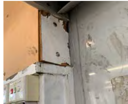
Damaged wall finished and exposed timber panels.
