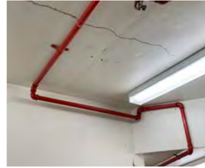
Cracks noted in concrete soffit.
