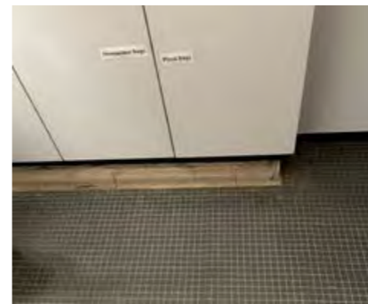
Skirting/ finish to plinth missing. Significant cracking visible.
