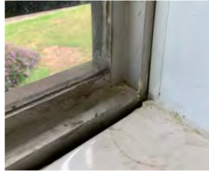
Seals/Caulking on external windows crumbling, and some areas where there are open gaps between wind frame and tiled sills.
