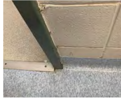
Room G32 - Vinyl pulling off walls in some areas
