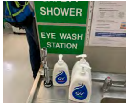
Non-compliant eye wash
