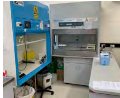
Non-compliant positioning of Fume Cupboard and Biosafety Cabinet. Room G10.
