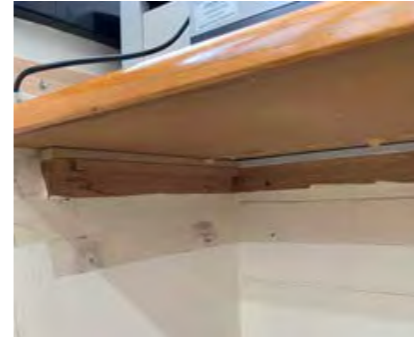
Exposed unfinished timber to most joinery.
