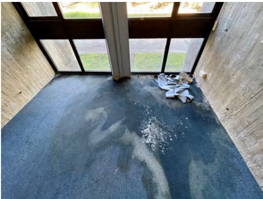
Water ingress at building façade
