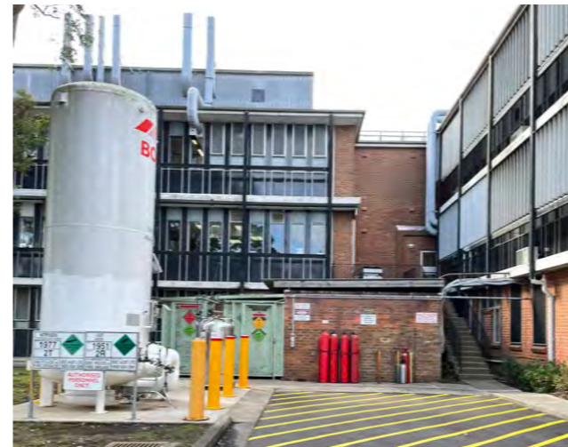
Image: gas storage
