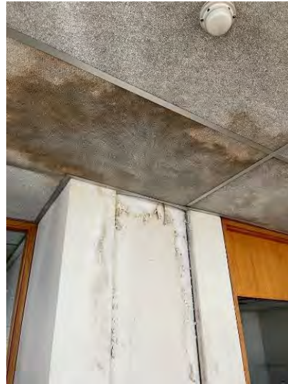
Extensive water damage at internal columns
