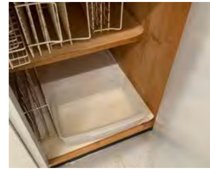
Exposed timber in underbench cupboards.
