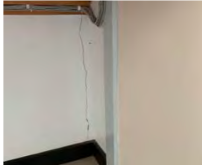
Cracks in blockwork wall. Structural review recommended
