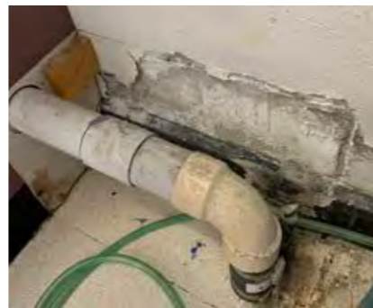
Water damaged walls and vinyl floors. Stained vinyl flooring with open joints. Exposed timber blocking.
