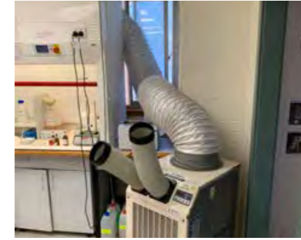
Inadequate air conditioning. Staff mentioned uncomfortable temperatures in labs during hotter days.
