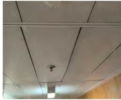
Perforated metal tiled ceiling are generally dirty and backing may be compromised exposing space to contaminants from ceiling space. Needs further investigation to confirm risks.
