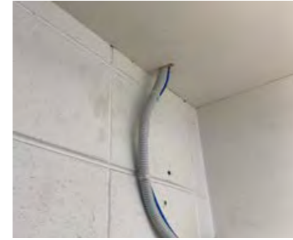
Walls generally not smooth or easily cleanable. Retrofitted services penetrations not appropriately sealed/finished.
