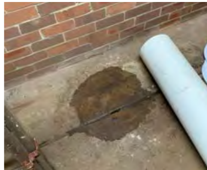
Recent evidence of moisture ingress from slab over
