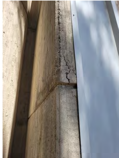
Cracking to external column
