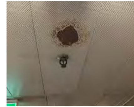
Damaged/stained ceiling tiles. Possible leak in above ceiling services.
