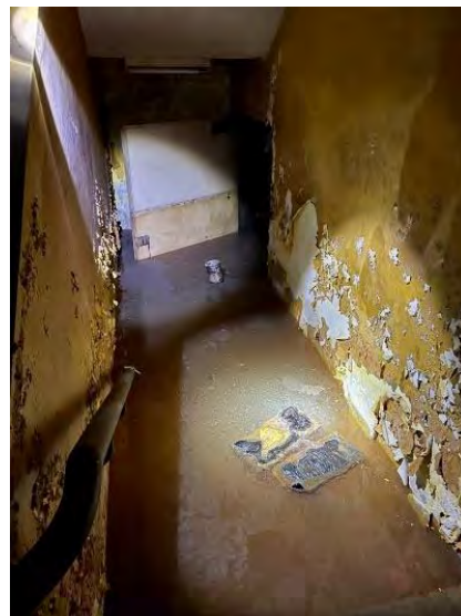
Standing water in stair cores
