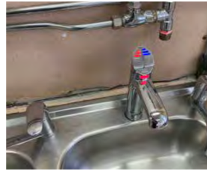
Junction at sink and splashback needs to be resealed.
