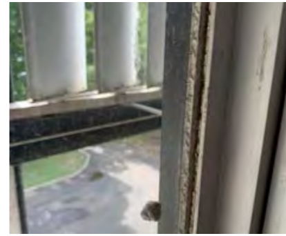
Seals/caulking to external windows crumbling
