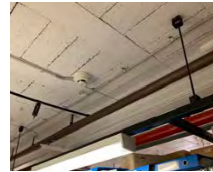
Evidence store ceilings generally exposed concrete planks with gaps, not generally smooth or easily cleanable.
