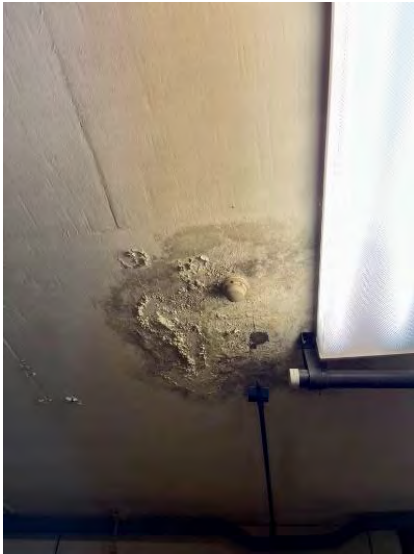
Evidence of likely reinforcement corrosion and concrete spalling at penetrations for services
