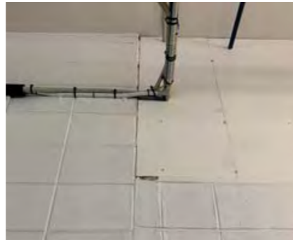
Painted blockwork walls and undulating surfaces not fully sealed and difficult to clean.
