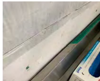
Splashback not sealed to walls.
