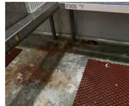
Coldroom floors rusted/stained, and generally whole room is in poor condition.
