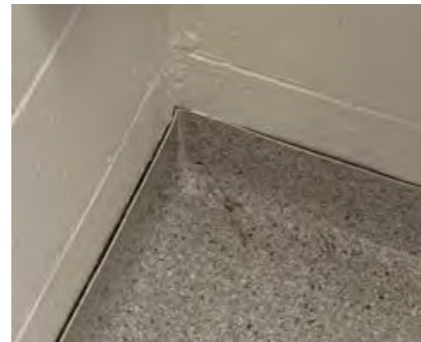
Coved vinyl skirting pulling away from wall
