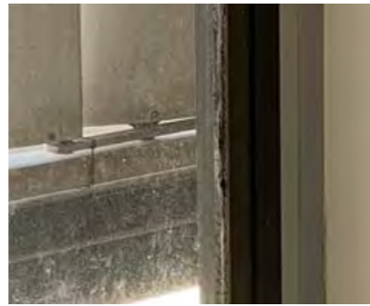
Seals/caulking to external windows crumbling.
