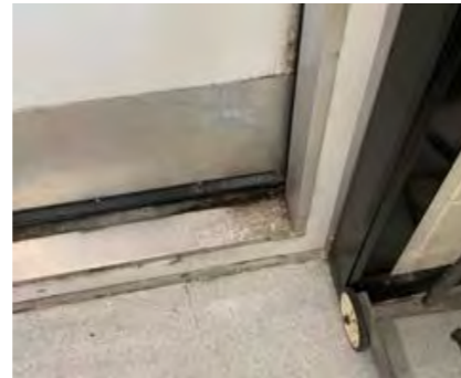
Door threshold into cold room, dirty and hard to clean.
