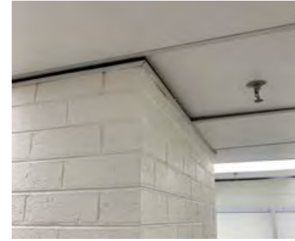
Large gaps at wall to ceiling junctions throughout
