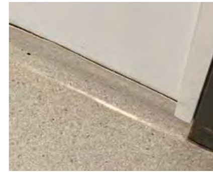
Vinyl coving pulling away from walls
