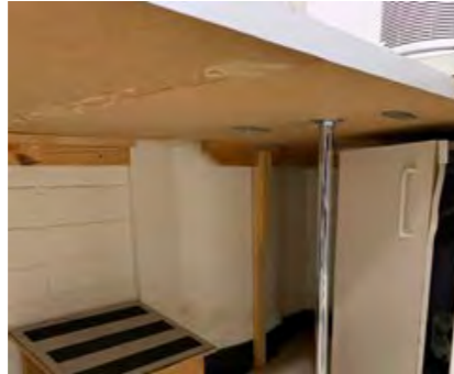
Joinery with exposed/unsealed timber
