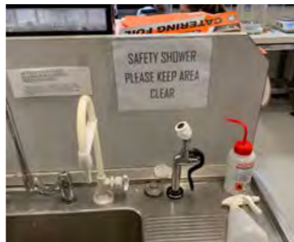
Non-compliant eye wash
