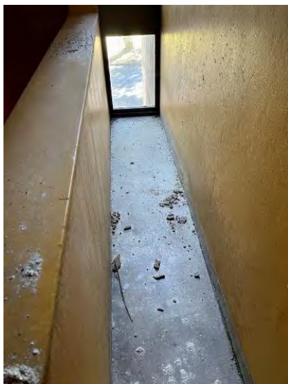
Spalling concrete from slabs over
