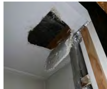
Damaged bulkheads and ceilings
