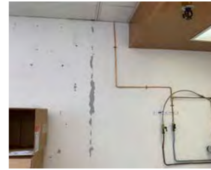
Damaged walls and timber bulkheads
