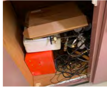
Exposed timber in all underbench cupboards.
