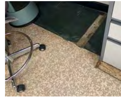
Damaged or missing floor vinyl at numerous locations.
