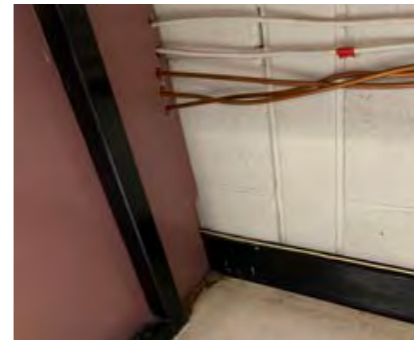
Numerous examples of services reticulation that have been retro fitted in-house, and not appropriately labelled or secured. This is typical of older laboratories where the flexibility and future proofing has not been considered in the original design.
