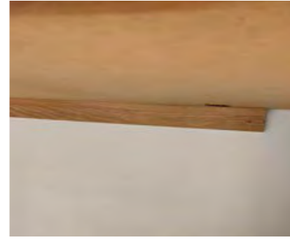
Generally unsealed timber exposed under benchtops.
