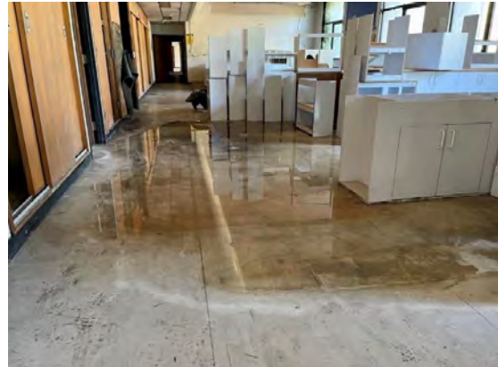
Ponded water throughout
