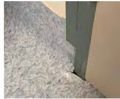
Vinyl coving pulling away from walls and not sealed junctions.
