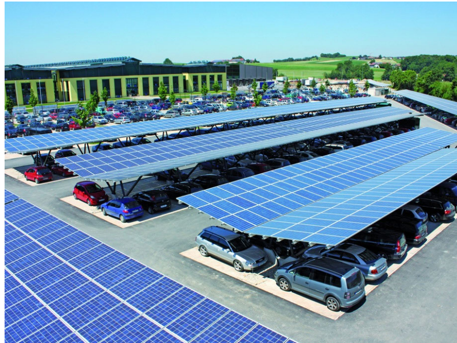
Figure 48: PV canopies shade car parks and provide renewable energy
